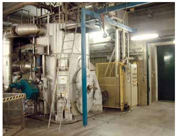
Armoured furnace for thermal disposal
