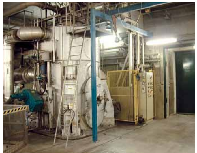
Armoured furnace for thermal disposal
